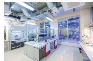
Monitoring the differential pressure, relative humidity/temperature and environmental CO 2 levels in laboratories where incubators are used
